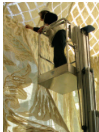
Left to right: Process of installing Janice Arnold's Palace Yurt in the Cooper-Hewitt's conservatory for the 2009 "Fashioning Felt" show; sketch of the north door, the site for the installation, the artist adjusting the felted fabric.
